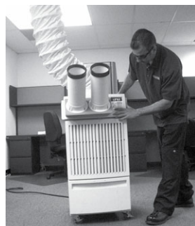
Portable cooling installation for temporary use in an office suite
